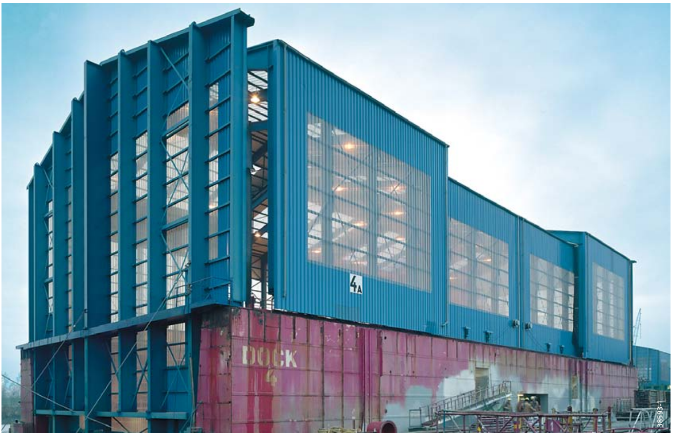
The roof sections of the dock can be opened smoothly
